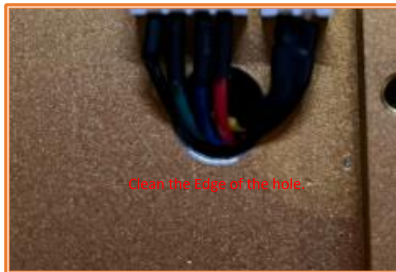
Figure 17: Use a file or sandpaper to smooth the edge of the hole.
